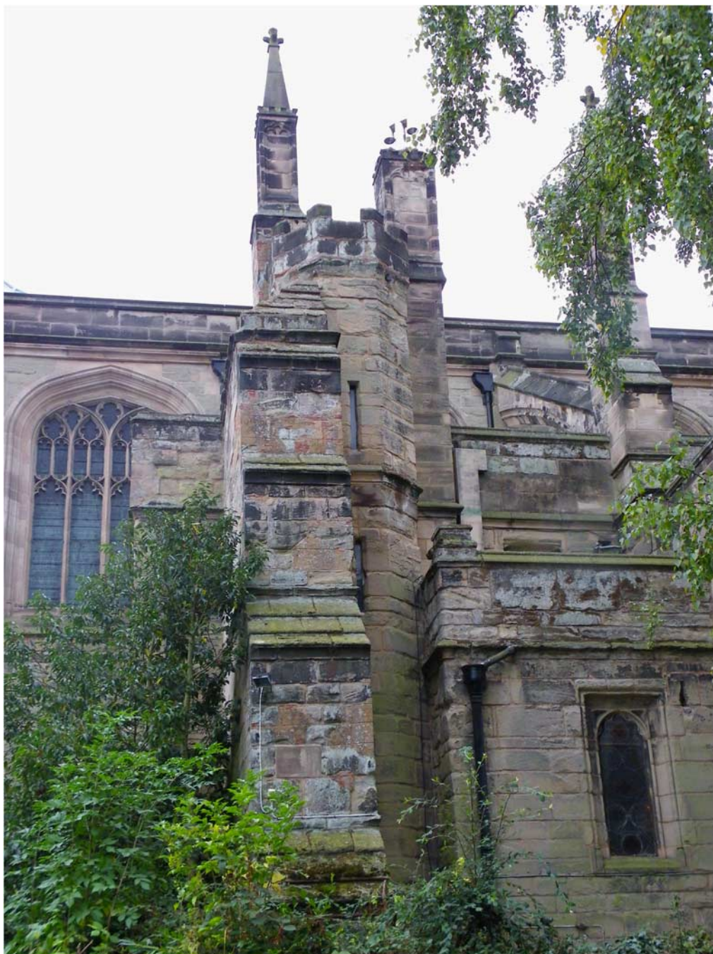
Fig 5. Exterior of the sacristy, showing a buttress, stair turret and chimney. Photograph: author
