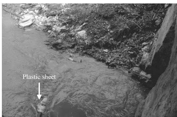
Fig. 3. Leakage in water pipeline tied with plastic sheet, Hyderabad old city, 2005.
