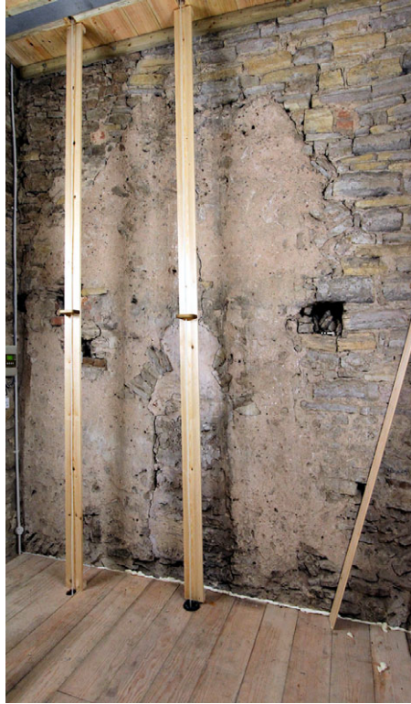
Fig 10. The first-floor chamber of the west tower looking towards the east wall. The blocked, rubble-headed opening is visible in the centre surrounded by light orange mortar. Above, the former pitched roofline is clearly visible, partially interrupted by later alterations. Photograph: authors.
