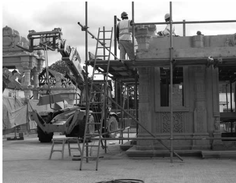
9 Construction of the Shiva shrine at the Sanatan Hindu Mandir, Wembley, London, 2011.
