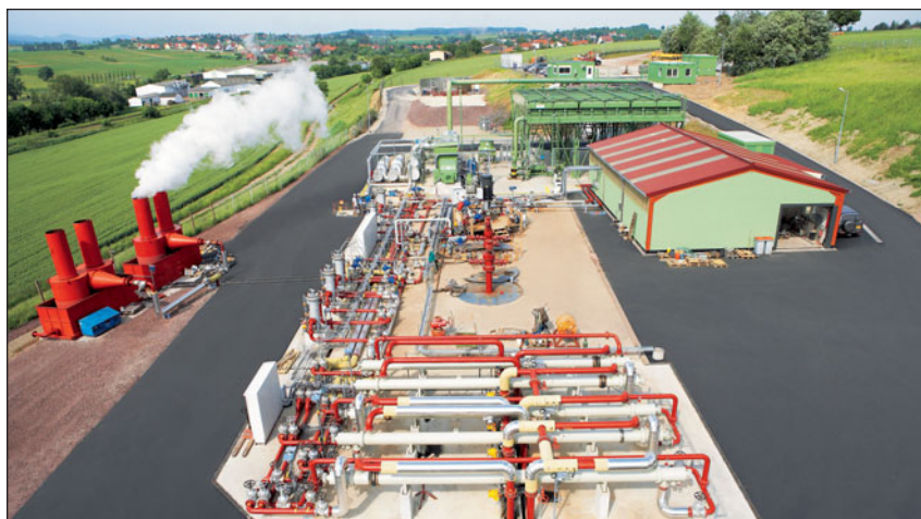
The European Geothermal Hot-Dry-Rock Project enhanced geothermal systems plant in Soultz-sous-Forêts, France, produces thermal energy from fractured crystalline rock for electricity. It also serves as a platform for basic research and testing. Photo courtesy of Groupeement Européen d'Intérêt Economique "Exploitation Minière de la Chaleur" (GEIE EMC).
