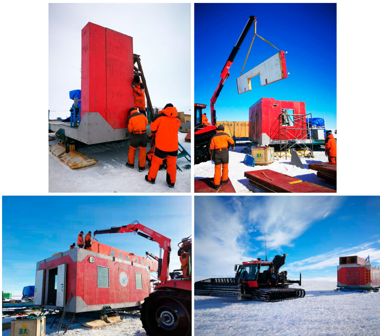
Fig. 12. ASDR assembly and transportation to the drilling site in the vicinity of Zhongshan Station, December 2018–January 2019.
