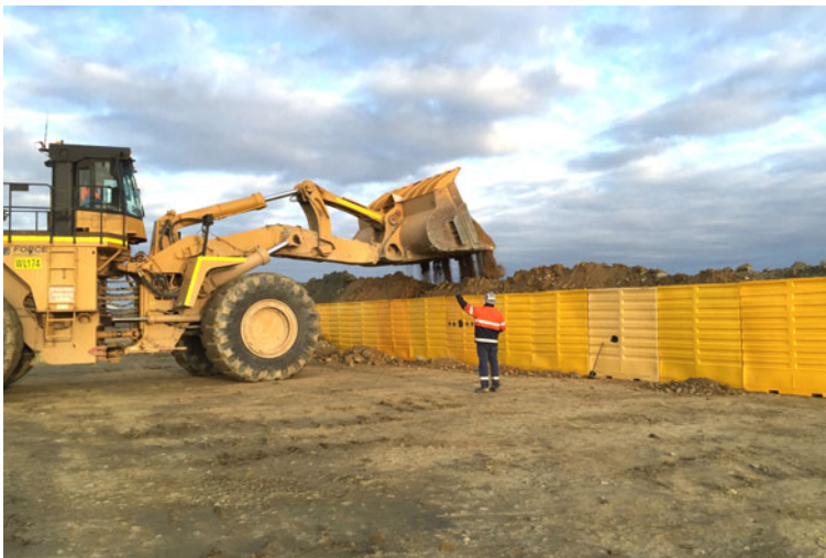
FIGURE 3. A loader placing rock material behind the units at the Edna May mine in Western Australia. The separate panels are linked together to form a vertical face behind which the top of the bund can be seen. Approximate dimensions can be estimated relative to the worker in the foreground.
