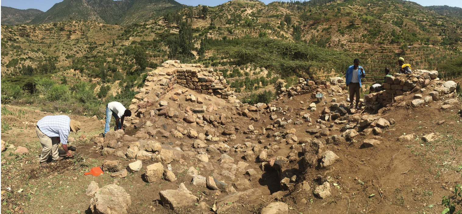
Frontispiece 1. A mosque of the mid twelfth to mid thirteenth centuries AD under excavation in the terraced landscape surrounding Harlaa, Ethiopia. Located at 1700m asl in the Afar region (midway between modern Addis Ababa and the Red Sea), Harlaa was a significant centre of population, production and trade from the mid first to mid second millennia AD. The site's importance is reflected in the archaeological evidence for its extensive exchange networks reaching into North and sub-Saharan Africa, across the Middle East and Indian Ocean, and as far as China. Investigations underway since 2015 have identified substantial and varied evidence for medieval Islamic communities at the site, including Arabic inscriptions and burials, and the site appears to have played an important role in the Islamisation of the region. Photograph © Timothy Insoll.
