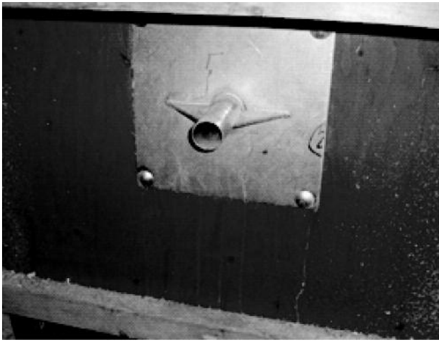
A pipe (nozzle) via which CO 2 is introduced through the wall into the barn at Farm A.
