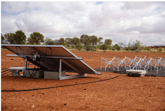
Figure 4. A Phase II long baseline tile. The batteries and BFIF systems are located under the solar panels.
