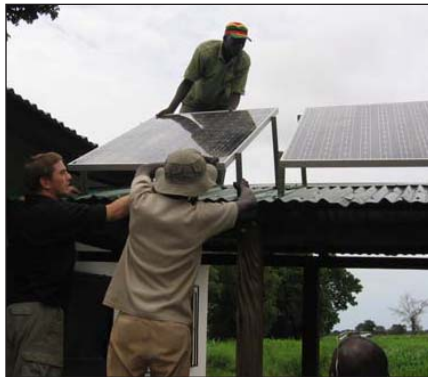
The Strathclyde team and the local contractor erect the solar panels on the roof of the village health clinic.
