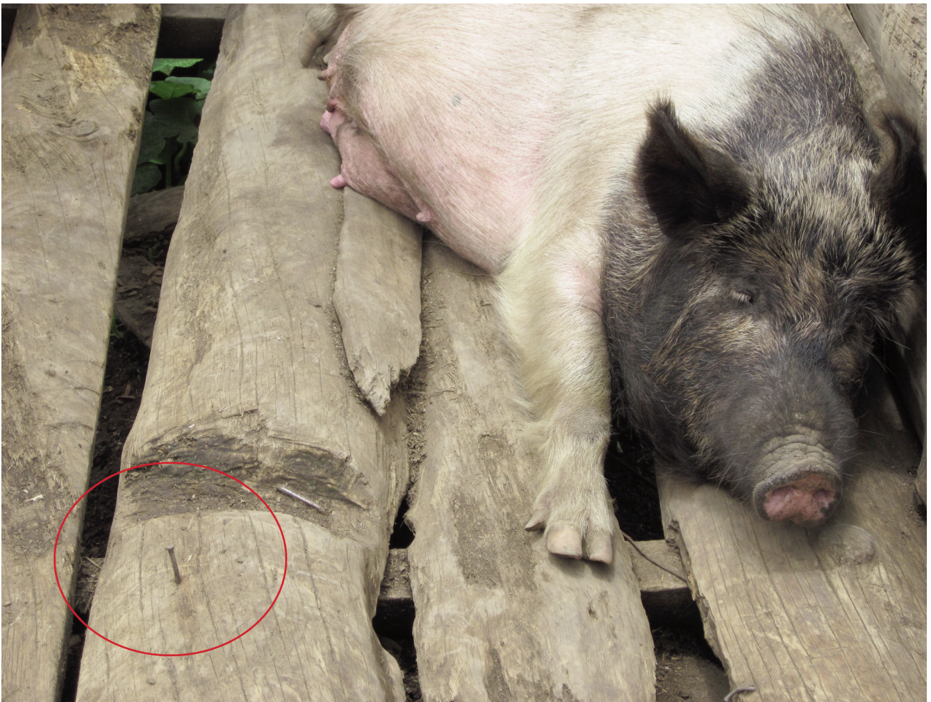
Floors of pen with a protruding nail and large gaps between the floorboards.
