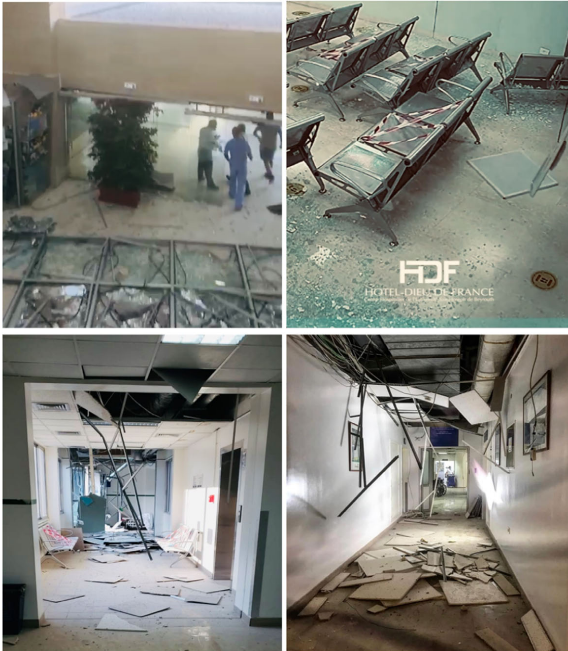
Figure 2. Shattered glass doors at the main entry, damage to the false ceiling, and power cut off.
