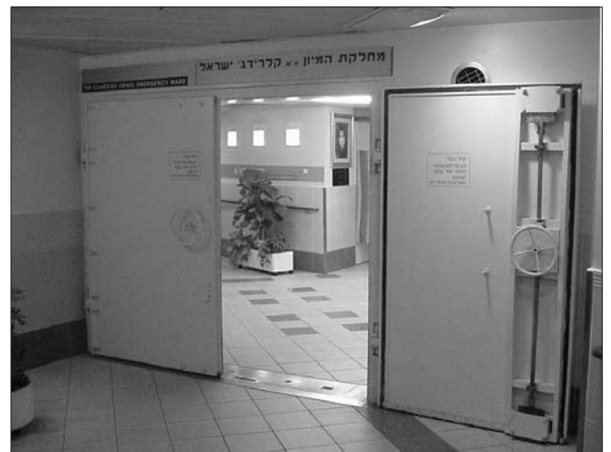
Fig. 2. The 3-cm steel doors to the entrance of the ED can provide a hermetic lockdown. The ED can function as a self-contained unit for 24 hours in case of biochemical attacks.
