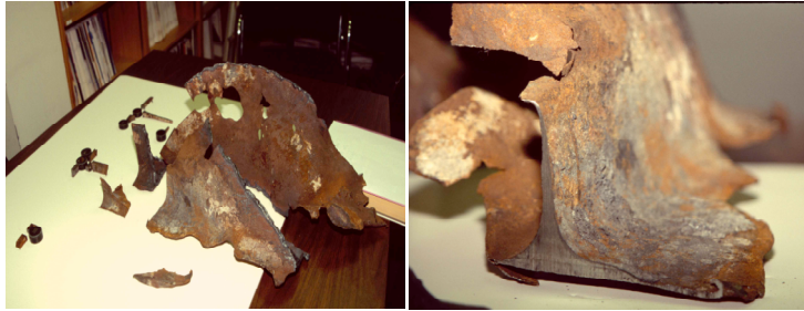
FIG. 1. Severely Eroded 1/2 inch wide flange beam from WTC 7.
