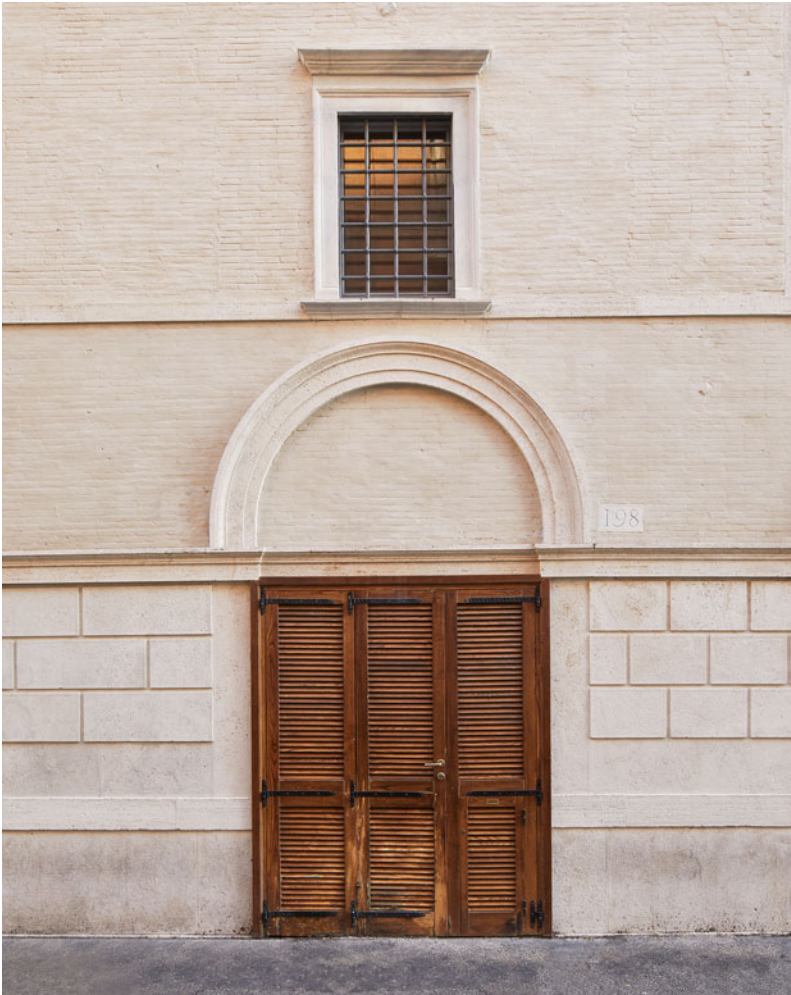
Figure 2. Palazzo della Cancelleria, Rome. Ornamental detail in travertine and brick. © Flavia Rossi.
